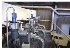
Oden P30R1 - "Steam Control" District heating plant, Mälarenergi AB, Västerås, Sweden
