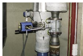
Oden P50R - "Hot water control" District heating plant, Tekniska verken, Linköping, Sweden
